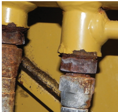
Figure 4: Corrosion migration to adjacent components
